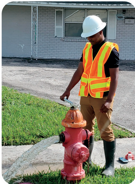
YEC Summer Internship - student interning with the City of Riviera Beach Water Utility Department flushing the fire hydrant
